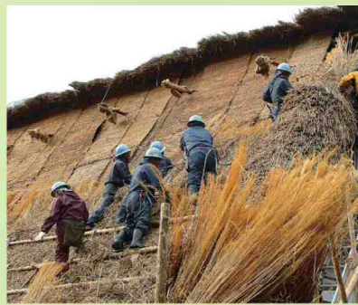
The roof thatching of gassho-zukuri is one of the seasonal events in Gokayama.
